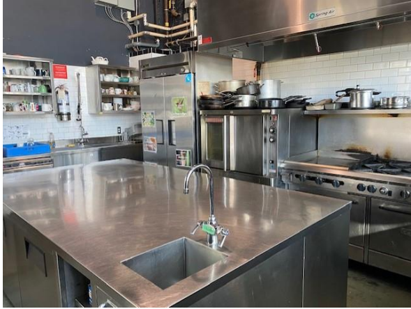
Commercial Kitchen Space
